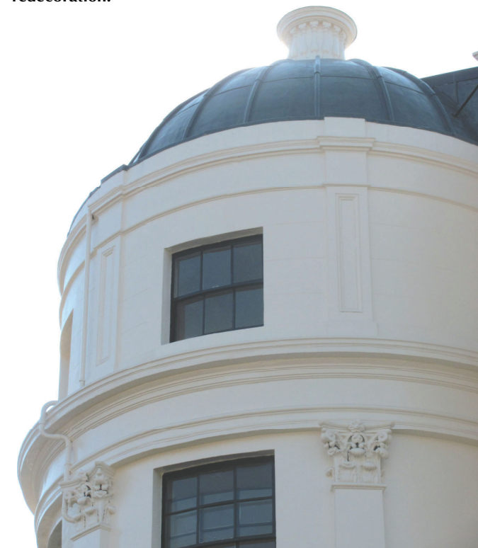
Completed external repairs, redecoration and re-roofing to 18th Century Georgian property in Victoria.
